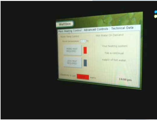
Wattbox control panel
